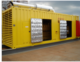
Typical external appearance of a transportable diesel generator set.
