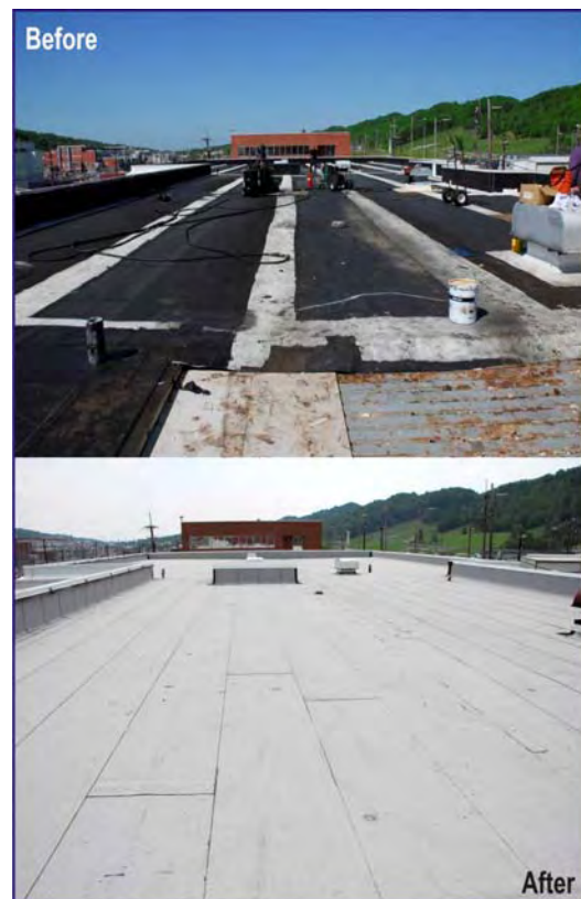
Figure A-11-2. Roof repairs on Building 9113 at Y-12. FIRP replaced 21,300 square feet of roofing on time and within budget.
