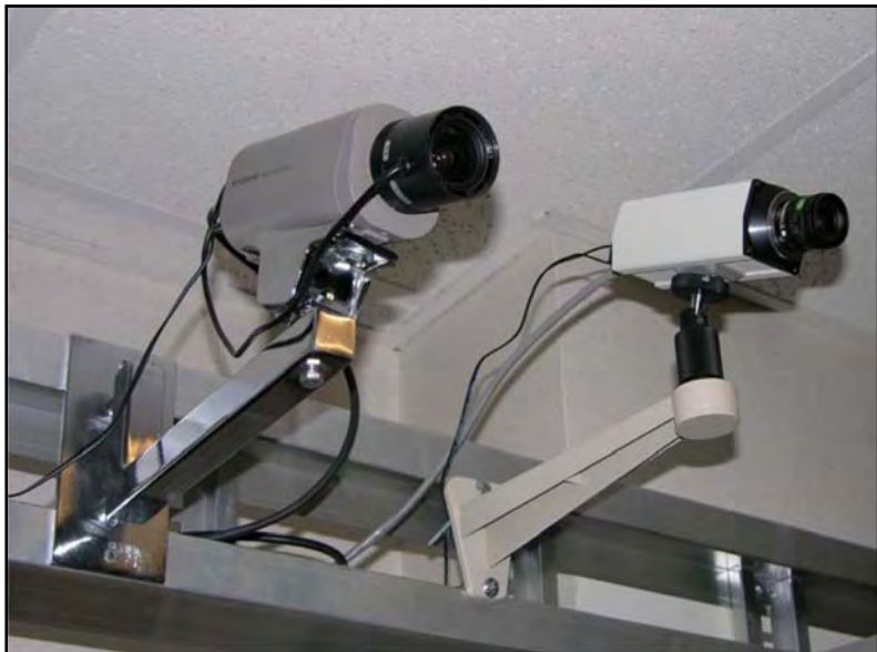
Figure A-13-4. Physical Security Systems provide security technologies deployed throughout NNSA sites.
