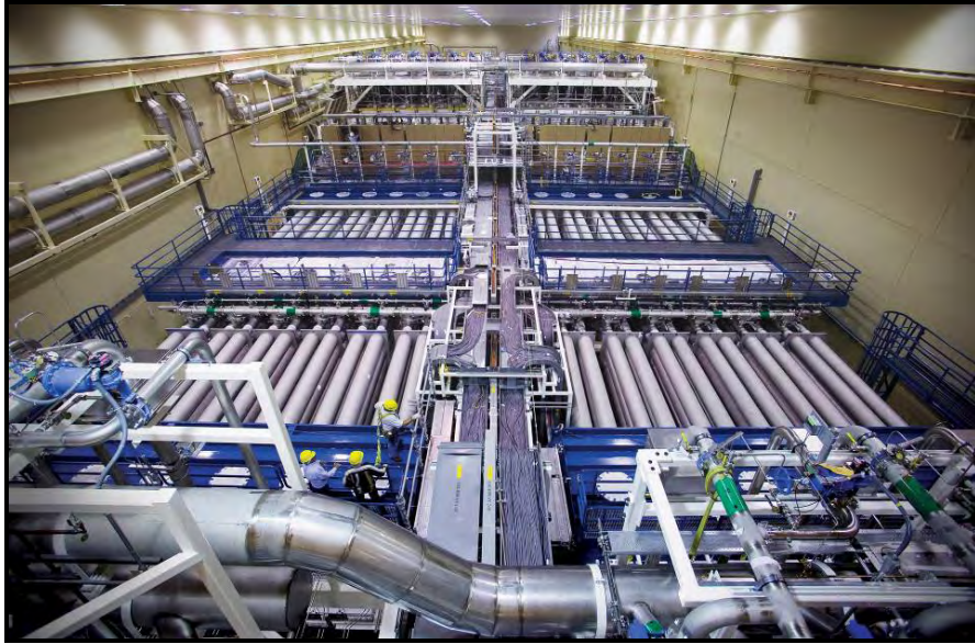
Figure A-5-3. One of two identical NIF laser bays, viewed from above. Each laser bay has two clusters of 48 beamlines.
