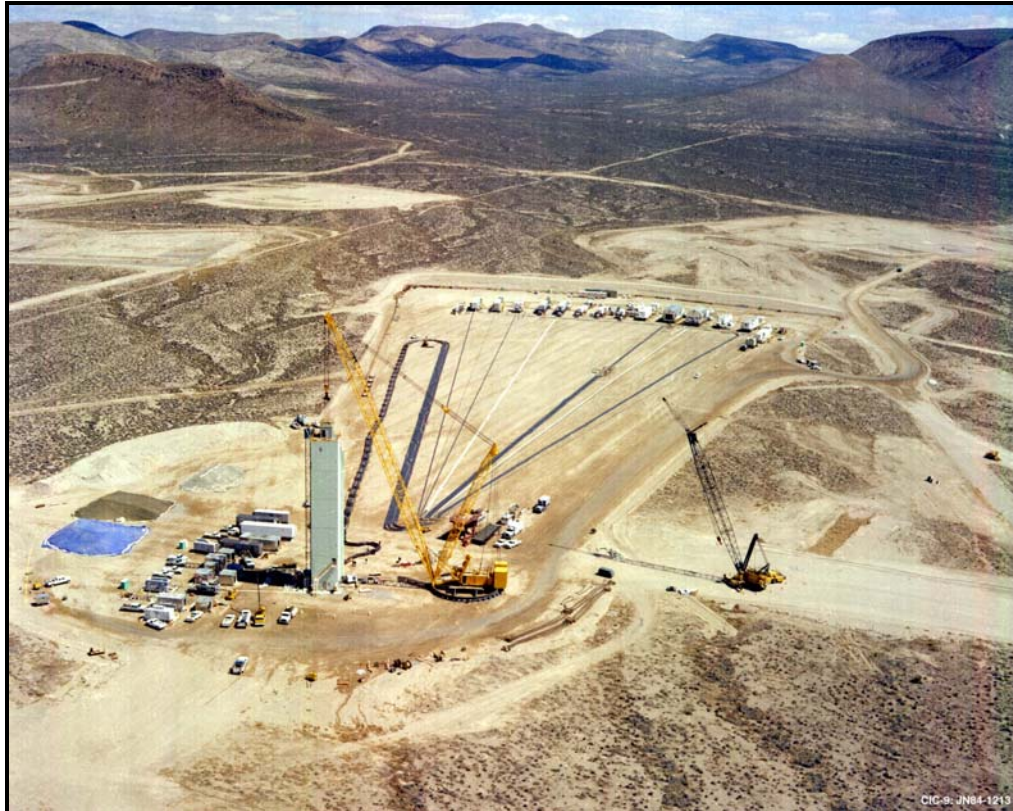
Figure 3-2. The test rack, suspended here by crane, is housed in a tower until the device is emplaced. The cabling is snaked between the trailers (outer edge) and the tower until lowered into the ground. Photo courtesy Los Alamos National Laboratory.
