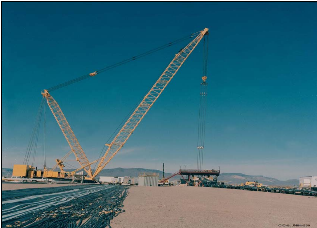
Figure 3-4. Crane lowering rack, device and cables into the test hole. Photo courtesy Los Alamos National Laboratory.
